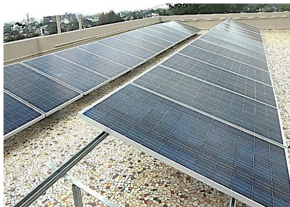
Solar Rooftop Solar panel
