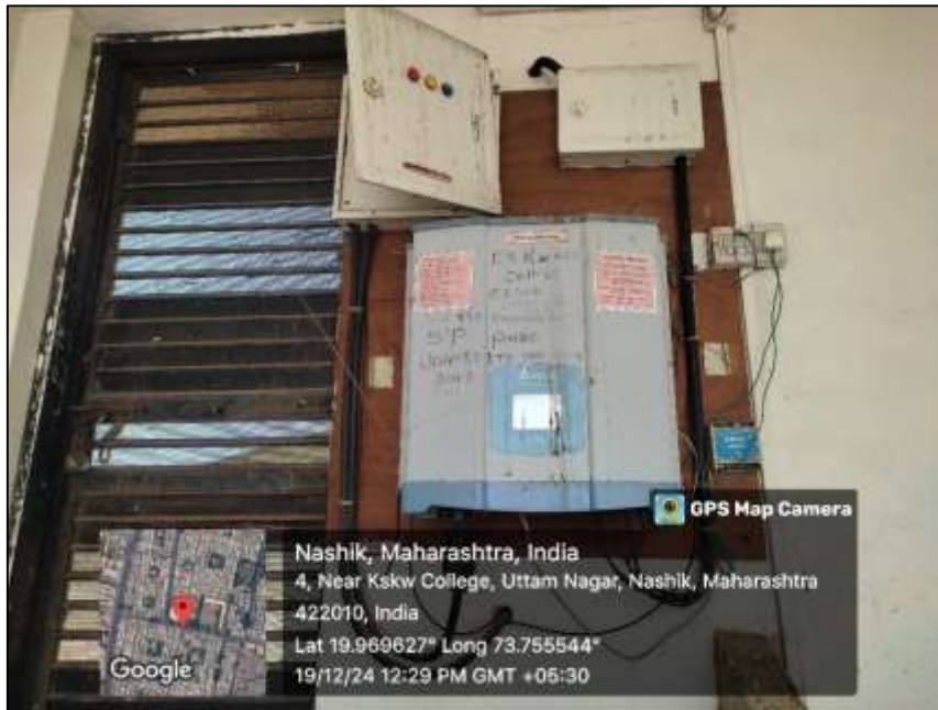
Solar on Grid Inverter (15.3KW)
