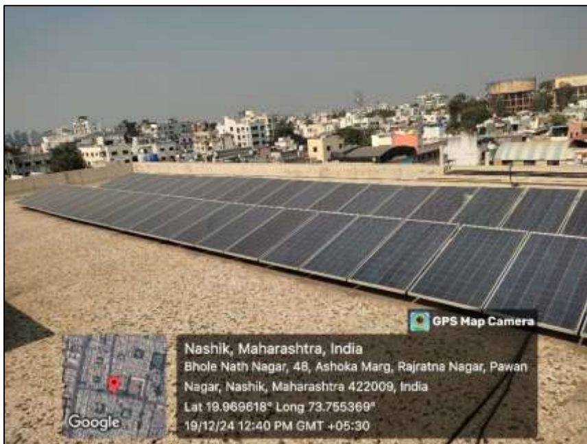
Rooftop Solar panel
