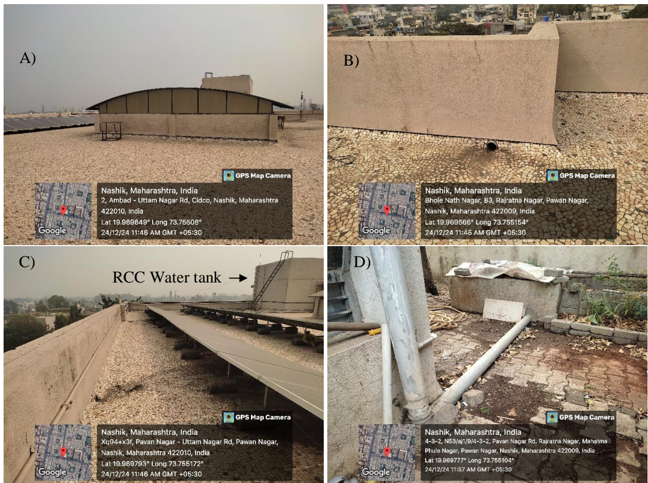
Figure A), B) & C) Terrace of the building with dome and water inlets to the water storage Figure D) Rainwater storage tank
