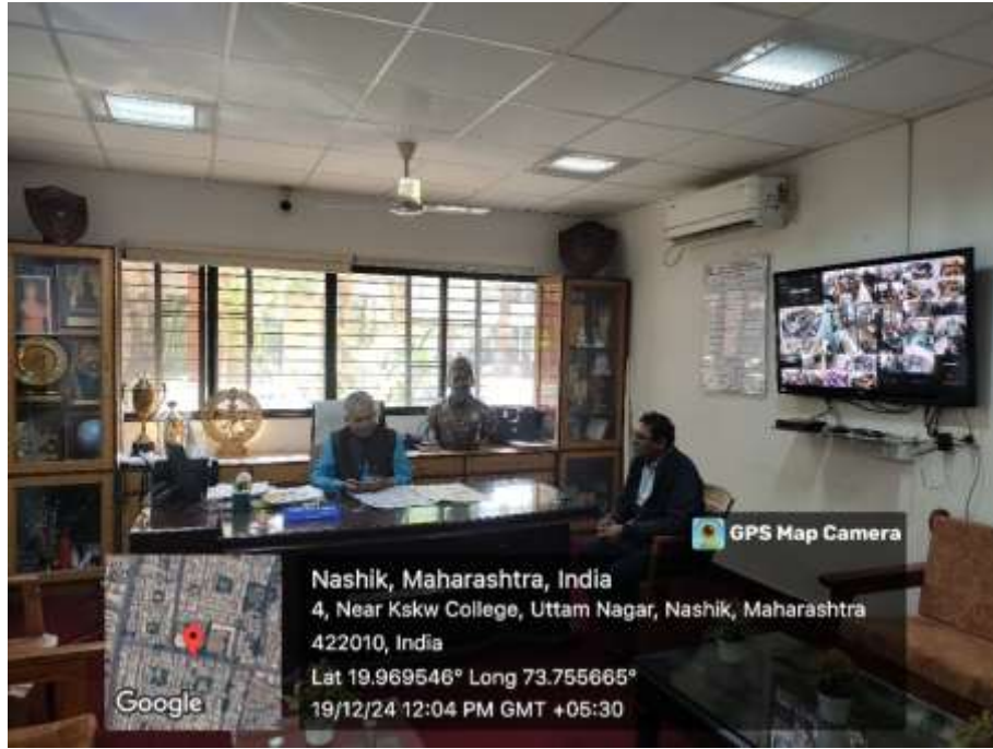
LED Bulbs in the Principal Office
