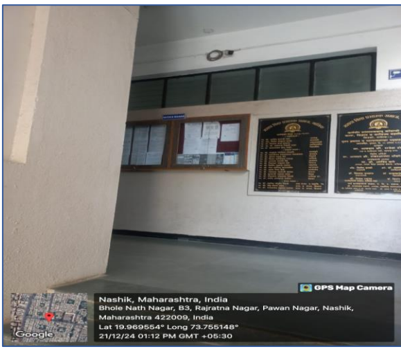
CCTV At First floor of New Building
